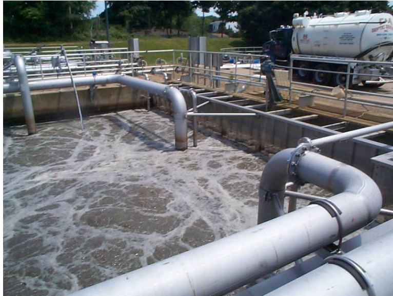
Figure 18 LinPor-CN™ Plug Flow Reactors at Westerly RI USA
